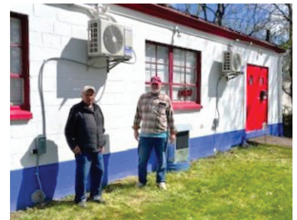
John R Fox Post 631 needed some help getting HVAC in their upstairs hall. AL members Ed Karlis & Steve Baumann as well as SAL member Devin Dickman (not pictured) stepped up and got it done with two new units. Now they have air conditioning and heat! -Story submission by Jerry Perry
